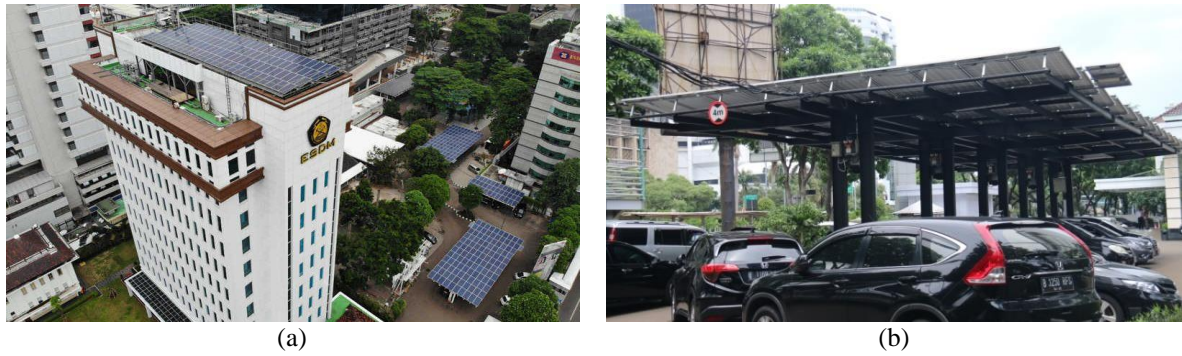
Figure 7. (a) Location of solar power plants of Setjen KESDM; (b) Installation method of solar power plants on the Setjen KESDM carport.
