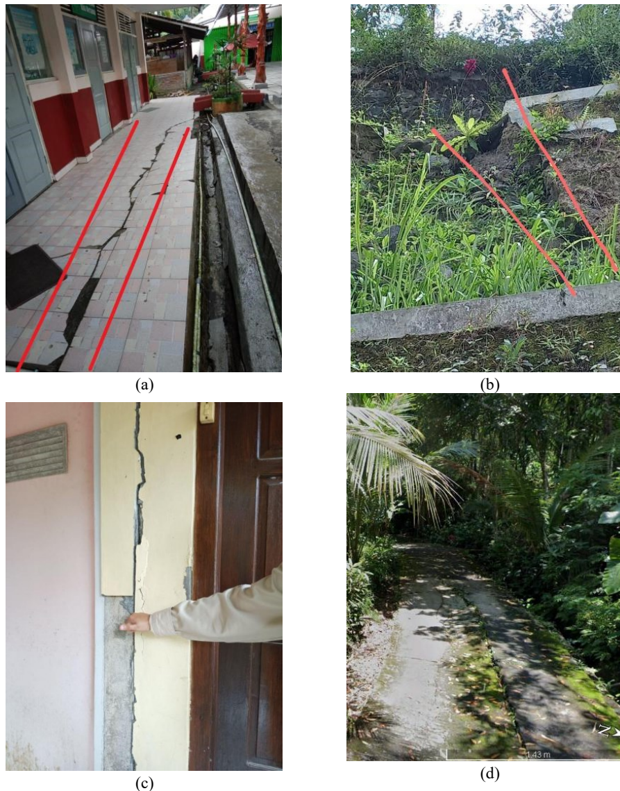
Figure 1. Cracks that occurred due to ground movement (a) cracks in the building of SMP N 1 Samigaluh, (b) cracks in the roadside wall, (c) cracks in houses, (d) cracks on the road.
